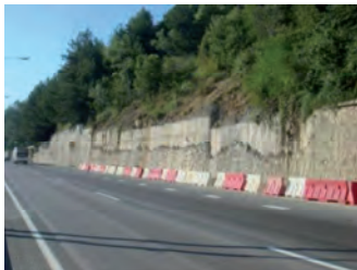
Figure 3. Upper retaining wall in Adler district (the 196th km) in the accident technical condition
