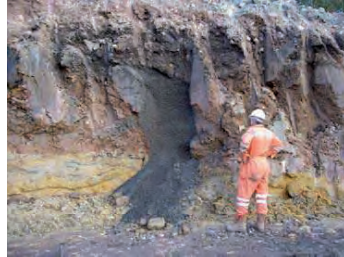
Figure 1 Shallow test shaft located during an earthworks operation near Tefford, UK. Note: the capping of overlying made ground and the shallow depth the shaft was taken to.
