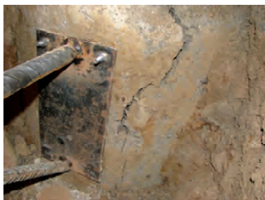
Figure 8. Cracks in the test pile located beneath the pile cap
