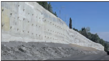
Figure 1. Pile anchor landslide protection structure at the interchange in the area of the city of Sochi
