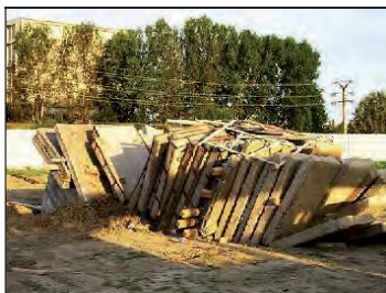
Figure 7. Collapse of the concrete slabs.
