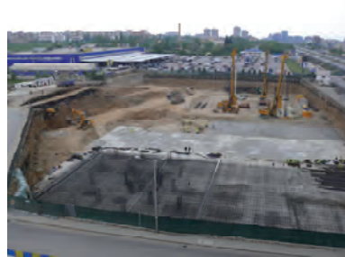
Figure 2. Pile construction beneath the high-rise footprint and raft construction in the low-rise area
